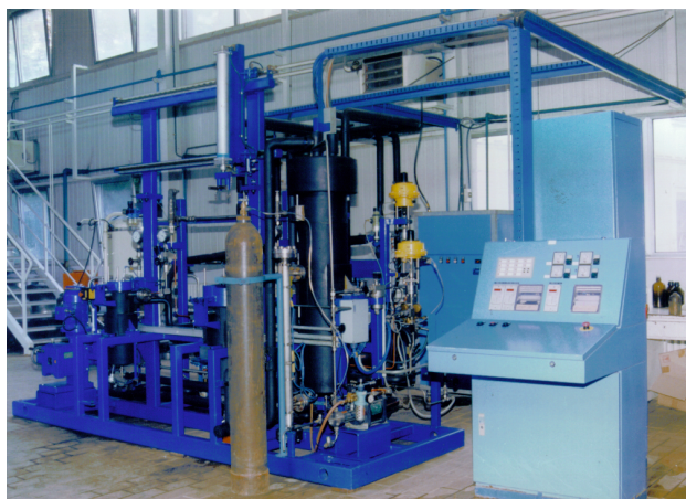
Fig. 2. SCGE pilot plant (Uhde GmbH, Germany)
